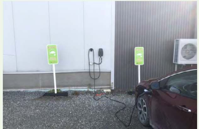
Electric vehicle charging station at our Val-d'Or office
